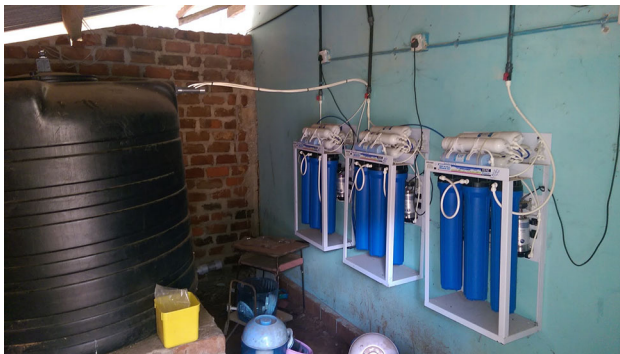
Fig. 3 A medium-scale RO plant
